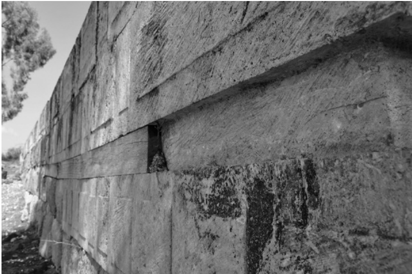
Figure 41: Photo of the Reconstructed Southwest Corner of the T-North Podium at the Present Site of Tel Dan Illustrating the Ashlar and Beam Construction Technique (photo by J. Greer).
